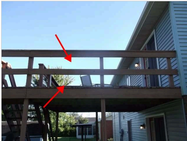
Deck's guard railings are climbable by a small child.
