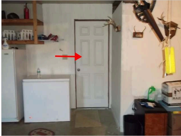
The garage mandoor into the home is not fire-rated.
