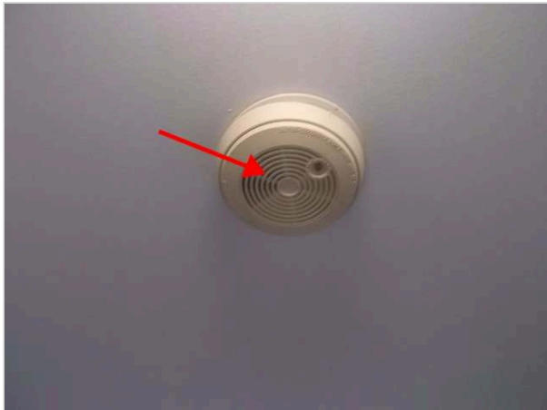
The installed smoke detectors are more than 10 years old (original) and should be replaced.
