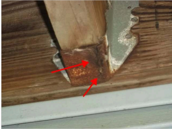
Deck's NE corner joist hanger is rusted and cracked.
