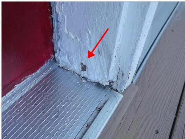
Rotted wood trim was noted outside the front entrance door.
