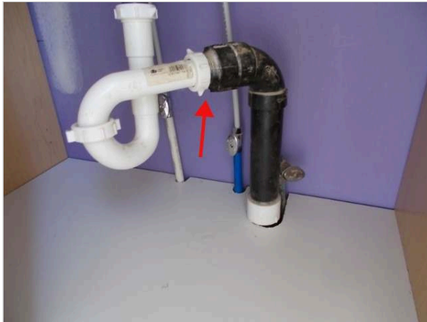
Leak was noted at the master bathroom sink's drain pipe.
