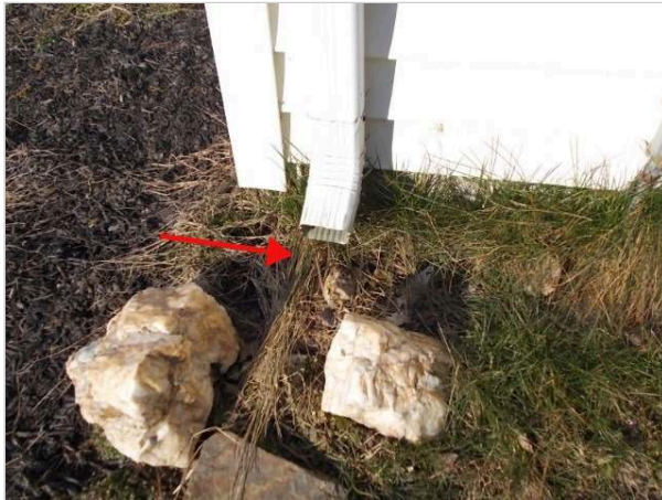
Multiple downspouts discharge along the home's foundation.
