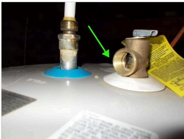
The water heater's T&P valve lacks its required discharge pipe.
