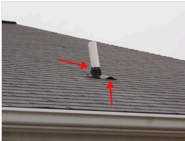
A partially torn and lifted boot was noted at the main roof's SE corner plumbing stack vent.
